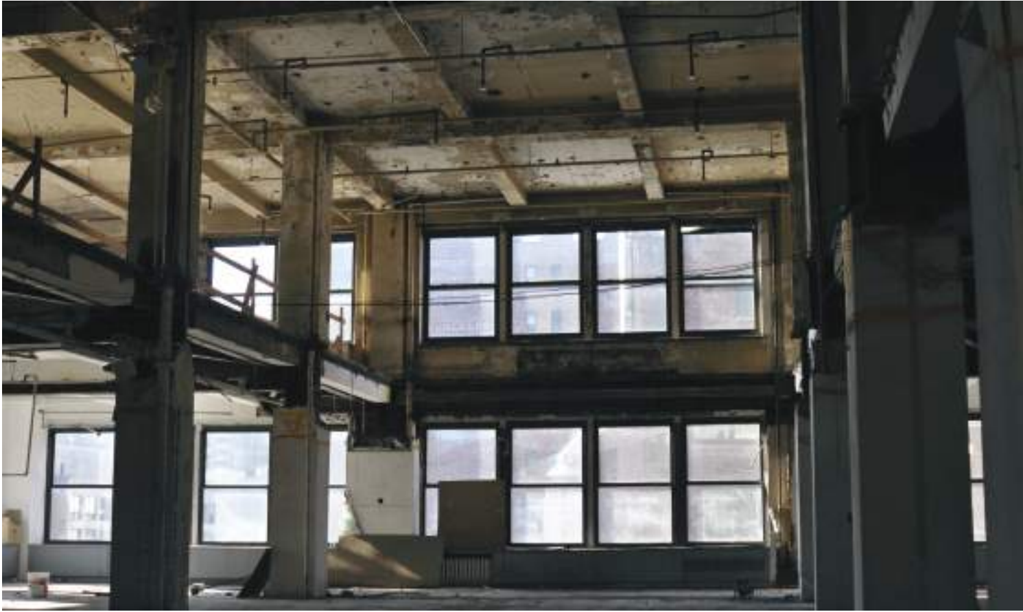
Demolition begins for the National Opera Center. Photo on page 24 is courtesy of OPERA America, the photos on page 25 are by Jeff McCrum.
